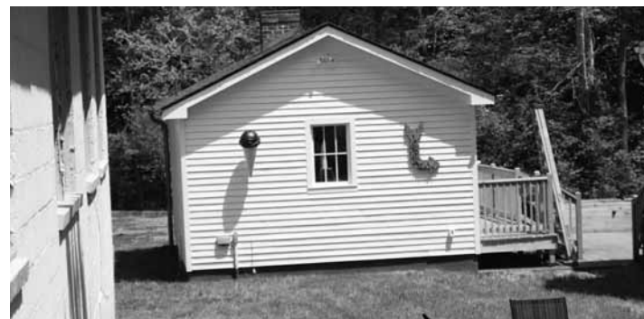
Outbuilding that does not follow initial design approved by ARB, according to town manager Matt Lawless.
