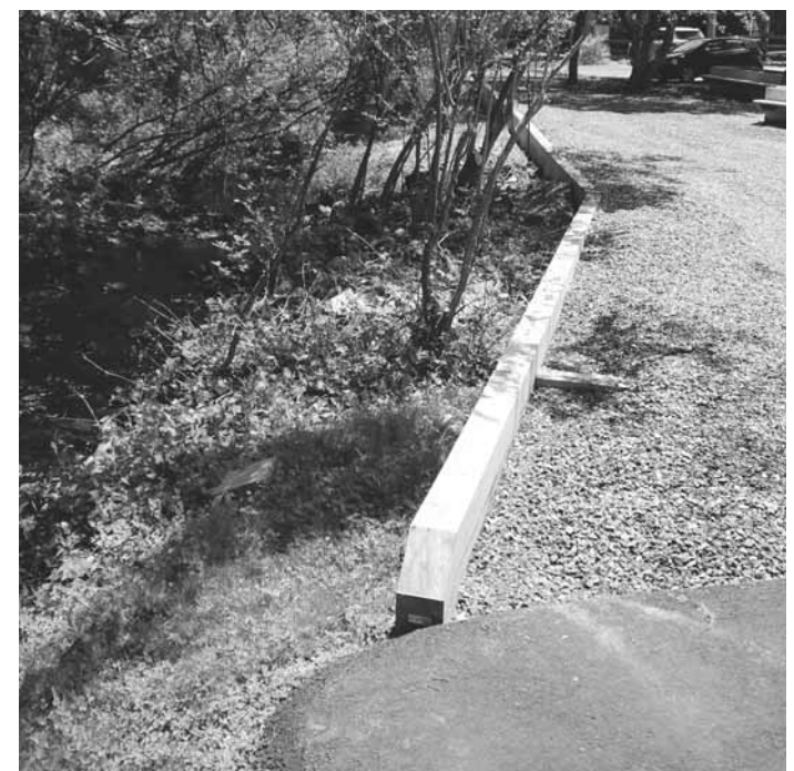
Unauthorized construction along Mink Creek, according to town manager Matt Lawless.
