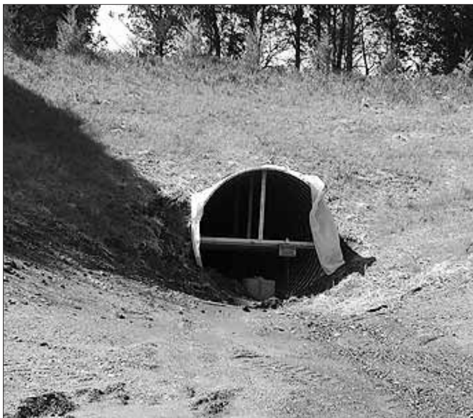
Virginia Vermiculite is digging a tunnel under Rt. 22 so that the mined mineral can eventually be transferred by conveyer belt rather than trucked.
