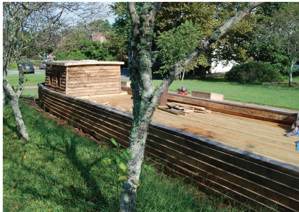
A replica of a "work boat" being constructed at Canal Basin Square in downtown Scottsville. This addition to the square marks a completion to the park by exhibiting not only a vessel that carried passengers but one that carried cargo on the historic canal.
