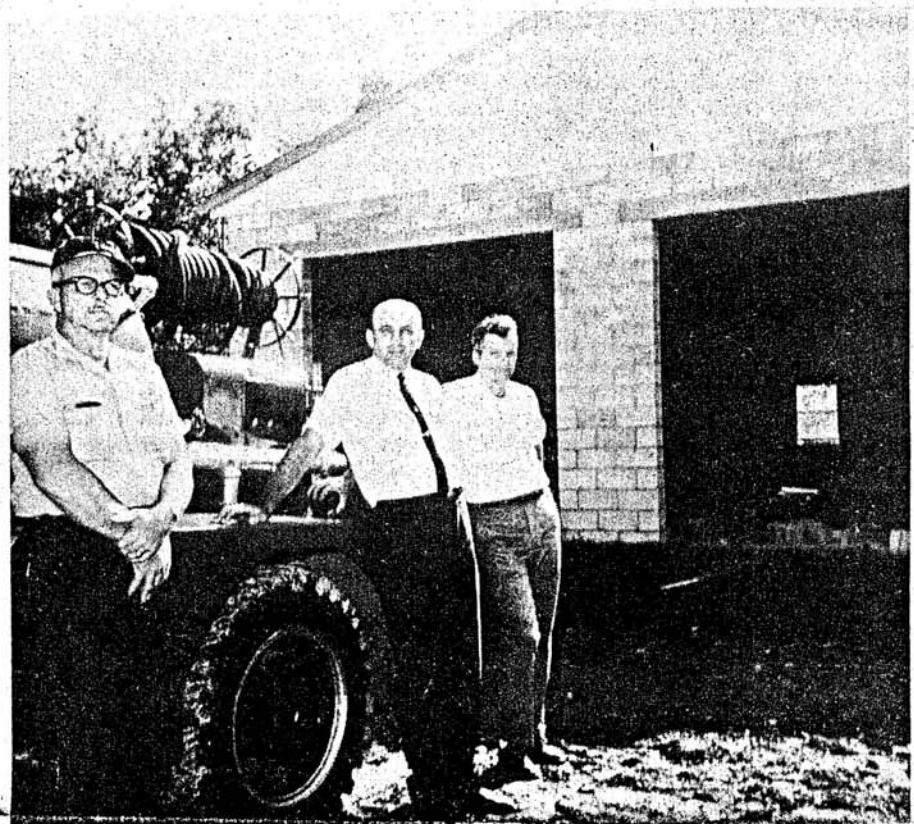
Standing in front of the new fire house, under construction, are Glenmore Fire Department members, left to right, L. L. Miles, Odell Ragland and Harold Snoddy.
