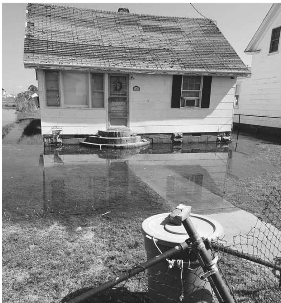
Typical low tide surrounds the foundation of the home.
