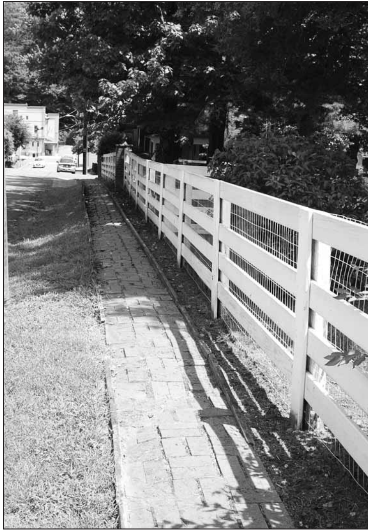
The sidewalk on Bird Street that needs to be replaced.
