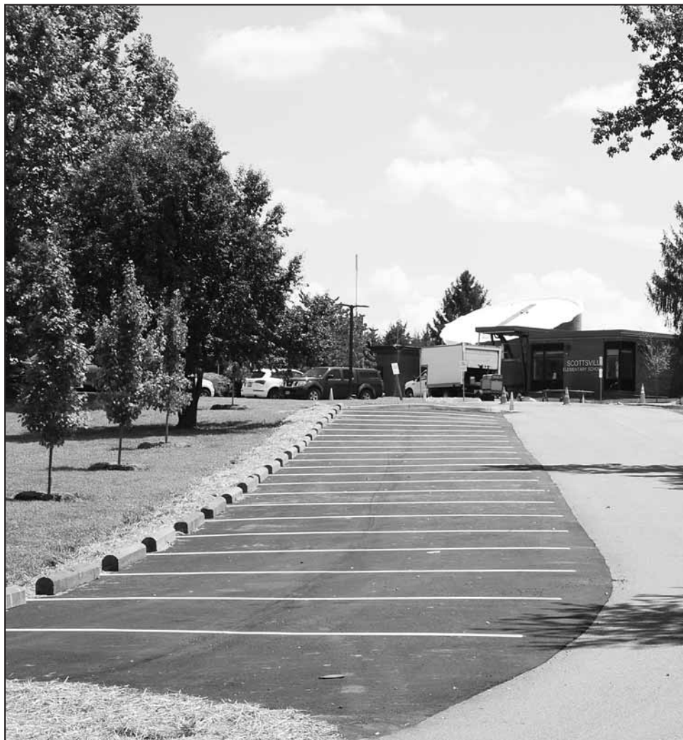
Work has been completed on much needed additional parking at Scottsville Elementary School.
