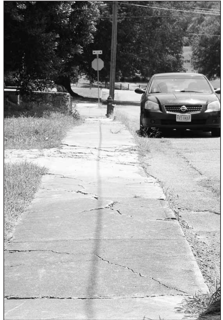
The sidewalk on Harrison Street, is in need of replacement.
