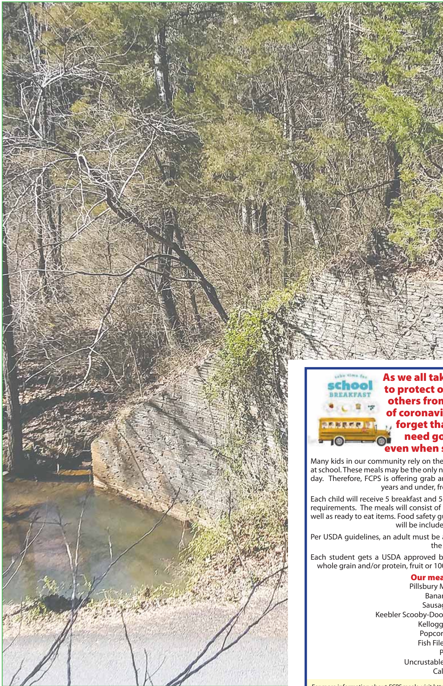
Watch Your Step! The northside abutment as seen from atop the southside abutment. There used to be a railroad bridge over Esmont Road up here. These abutments are made out of - what else? - soapstone.
