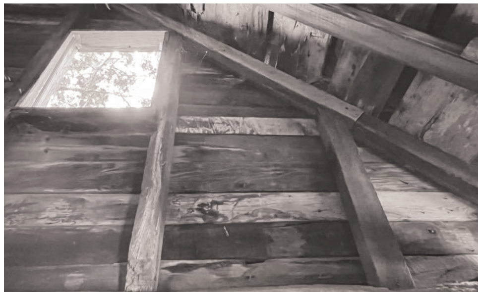
Looking up through the collapsed stairwell to the second-floor window; both joinery methods and materials used offer clues to the age of the structure.
