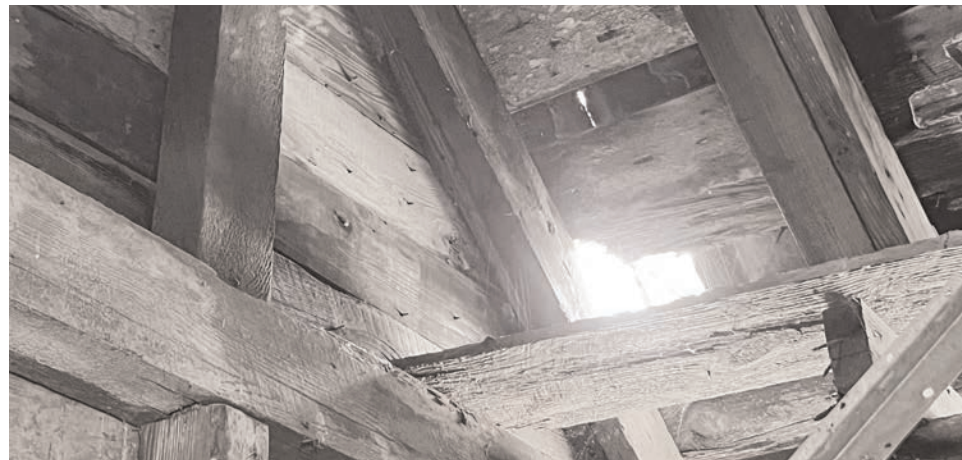
Both joinery methods and materials used offer insight into the structure’s age.
