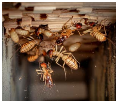
"Subterranean Termites at work—protect your home Today!"
